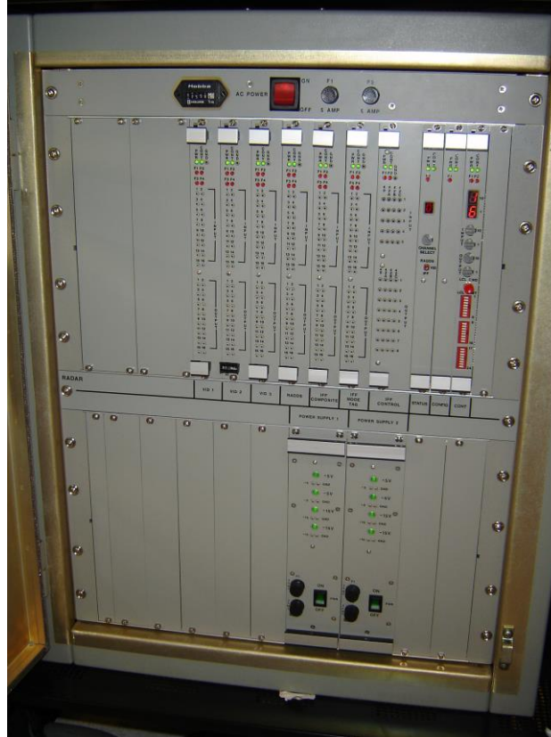
Figure 6-3: Radar Signal Distribution Switchboard (RSDS)
