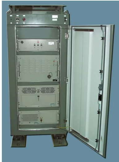
Figure 8-5: ES Processing Cabinet
