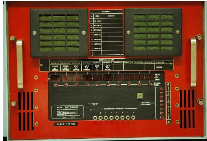
Figure 3-30: ACX-5A Red Voice Switchboard
