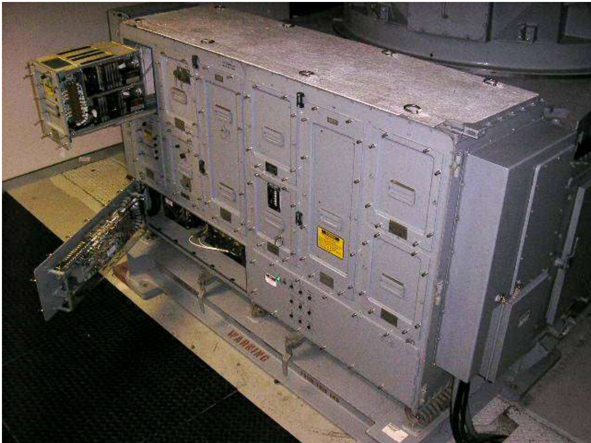
Figure 7-3: CIWS Electronics cabinet
