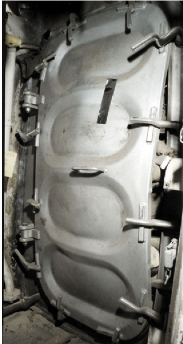
Fig 14-5. Damage to Fully Clipped Door Caused by Internal Explosion
